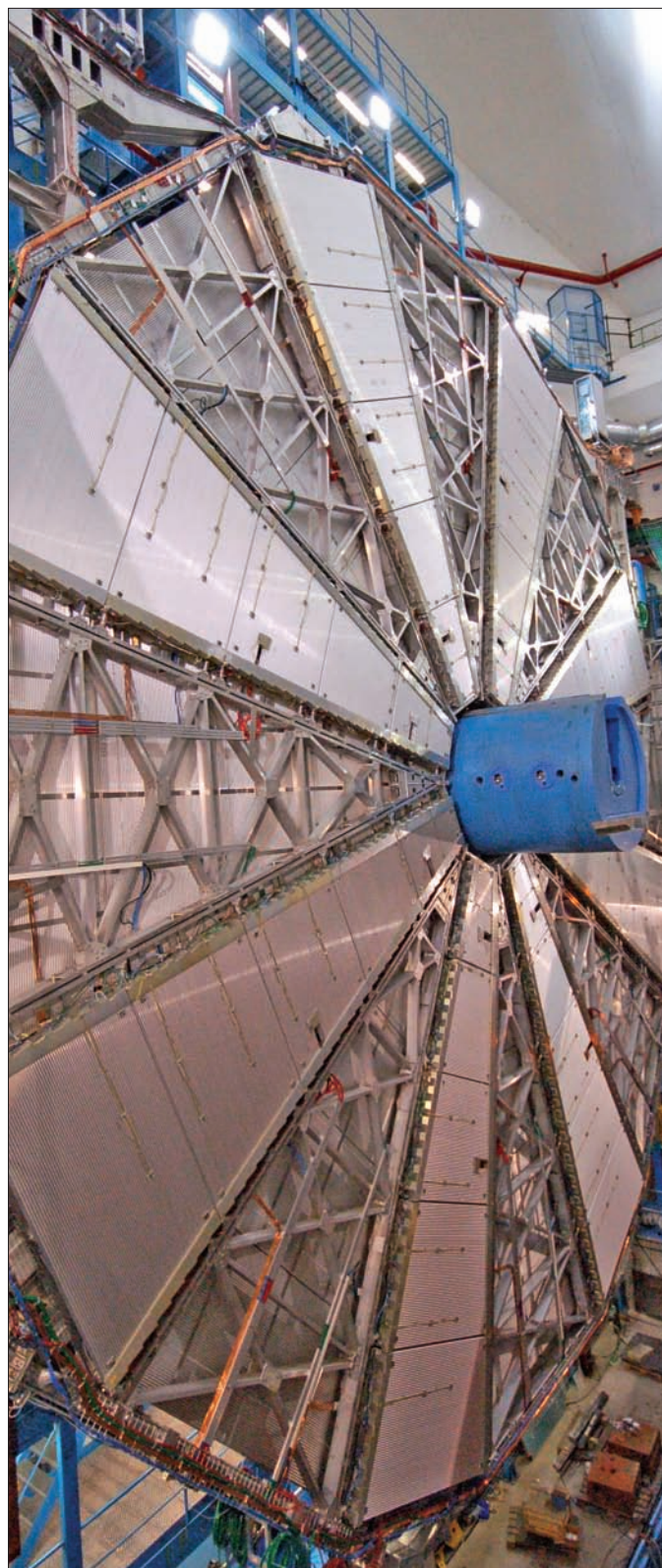
Fig. 6. The partially complete installation of MDT sectors in a big wheel for precision tracking. (Courtesy ATLAS Collaboration.)
